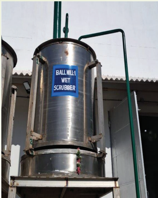
Wet Scrubber installed in pyroplant – MPMP
