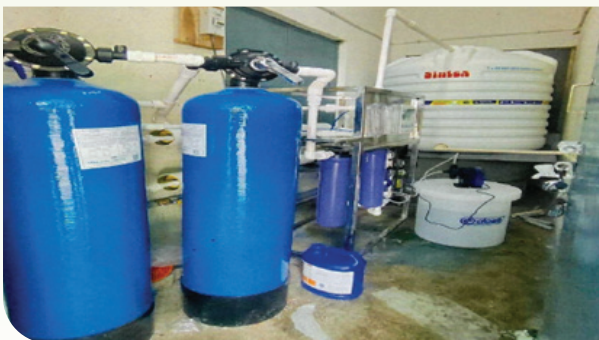
RO Plant – Panchayat Union Middle School, Vellaiyapuram
